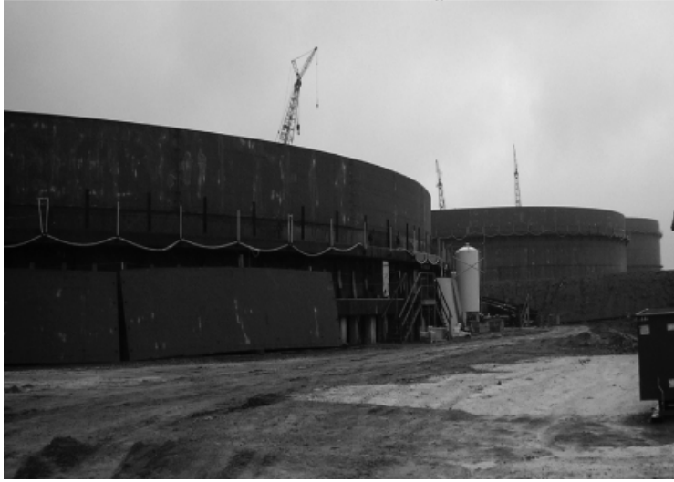
LNG Tanks Nos 1 through 3
