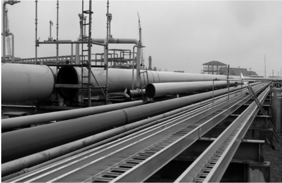
Pipeway from Marine Terminal
